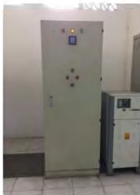
低压開閉器盤 (Outgoing Panel)
