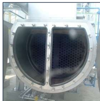
Waste Gas Boiler
