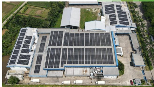
PT. Kanemory Food Service. 637kwp Sistem Pembangkit Listrik Tenaga Surya PV
