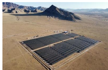
Tenaga Surya + BESS
