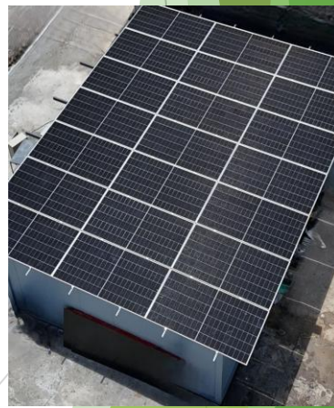
Solar panels on the temporary office rooftop
