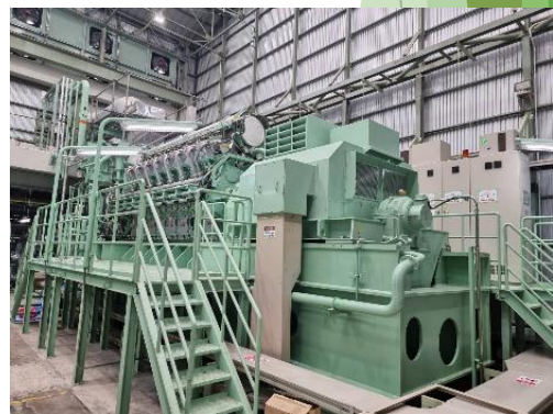
Cogeneration system (example in Thailand)
