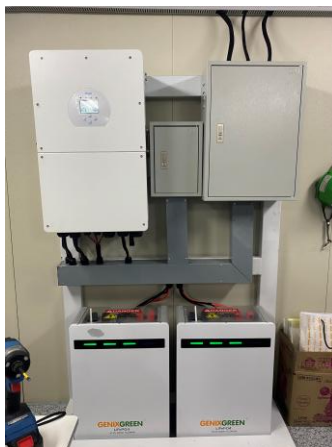
Power system equipment (battery & inverter)
