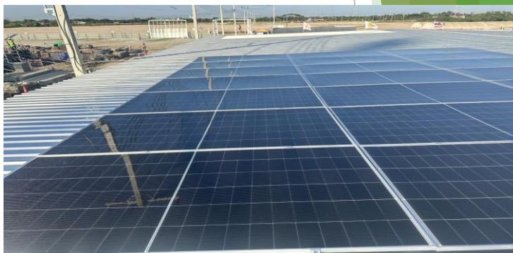
Solar panels installed on the construction site office rooftop in Thailand
