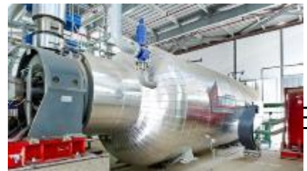
Waste Heat Power Generation
