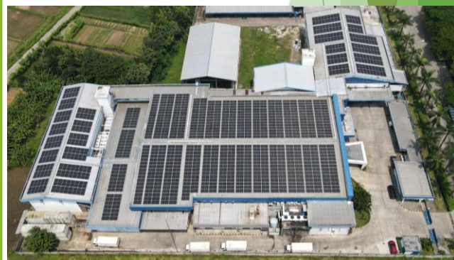
PT. Kanemory Food Service. 637kw solar PV system
