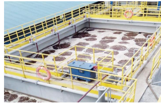
Image 2. WWTP Project Experience – Cilegon Area
