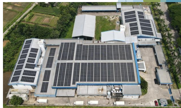
PT. Kanemory Food Service. 637kw Solar PV System
