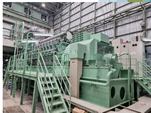
Cogeneration system (example in Thailand)
