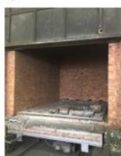
Inside of heating facility Brick design: Slow heating up / Quick heating down
