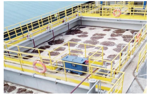
Image 2. WWTP Project Experience – Cilegon Area
