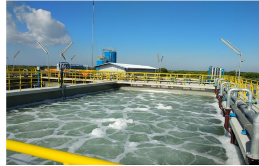
Image 1. WWTP Project Experience – Gresik Area
