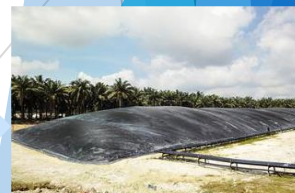
Bio Gas Power Generation
