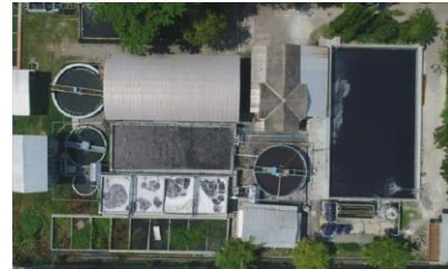
Instalasi Pengolahan Air Limbah (IPAL) Waste Water Treatment Plan
