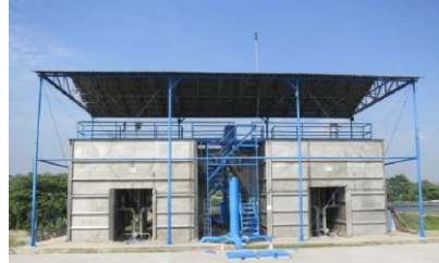
Pengolahan Air Bersih Water Treatment Plan
