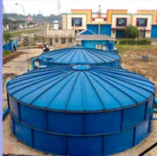
water treatment plan pengolahan air bersih
