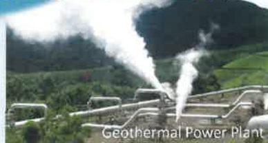
Geothermal Power Plant
