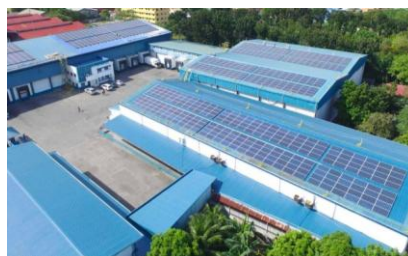
Client: Fast-Koldstor Capacity: 503.05 kWp
