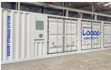
Nueva Era PV + BESS (PV 29,952kWp+4,386kWhBESS)
