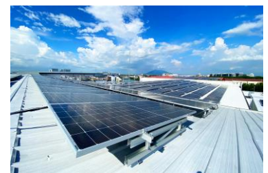
Clark C&I rooftop (PV1.297.10 kWp)
