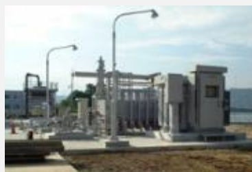
Electro chlorination systems
