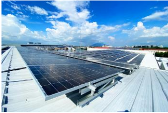
Rooftop solar power generation.
