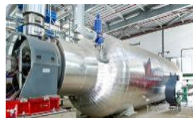
Waste Heat Recovery Power Generation
