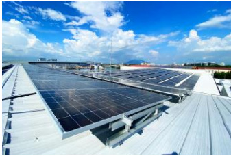
Rooftop solar power generation.
