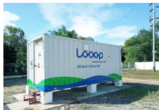
Container-type battery storage system
