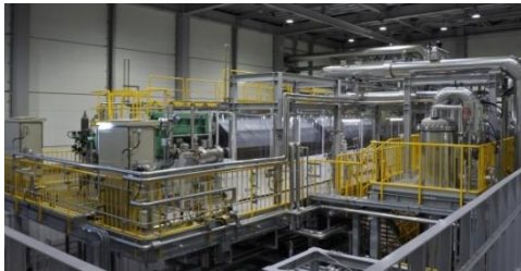
Large alkaline water electrolysis equipment
