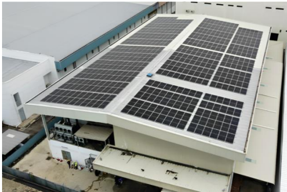
Solar power generation 265.98kWp (Malaysia)
