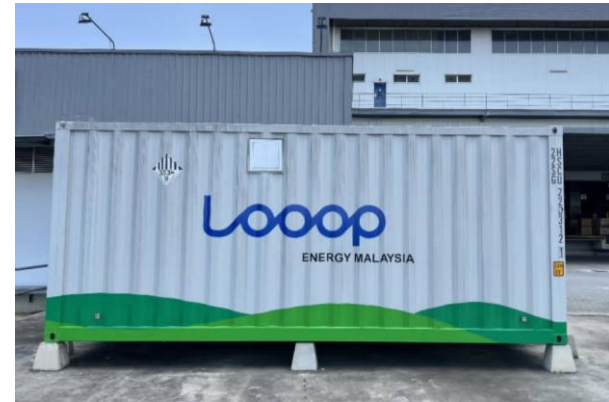
Storage battery (BESS) 500kWh (Malaysia)
